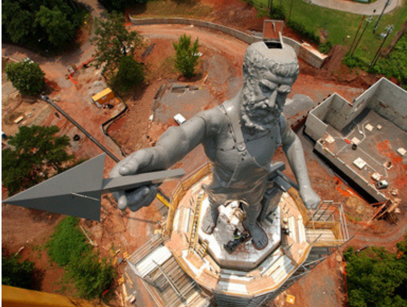
Vulcan as it looked like before being dismantled and renovated in 2001. The old tower on which the statue stood was also demolished in the process.
